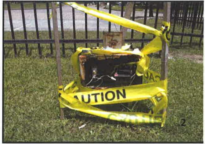
Bundy Lake Hazardous / Broken Gate Equipment
