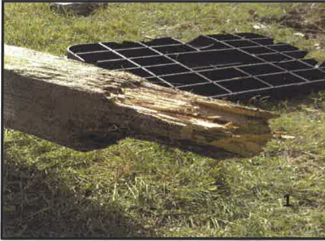
Rotted Light Pole by Bundy Lake Vault
